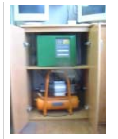
Plate 2.29 Processor and air compressor
