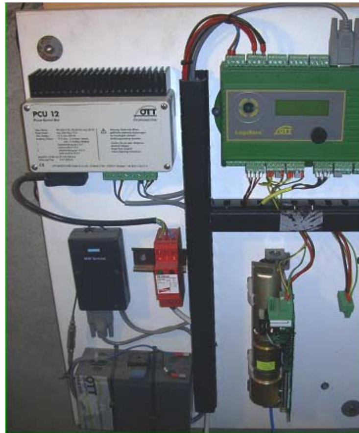
Plate 6.4 Tide Gauge Instrumentation (inside hut)
