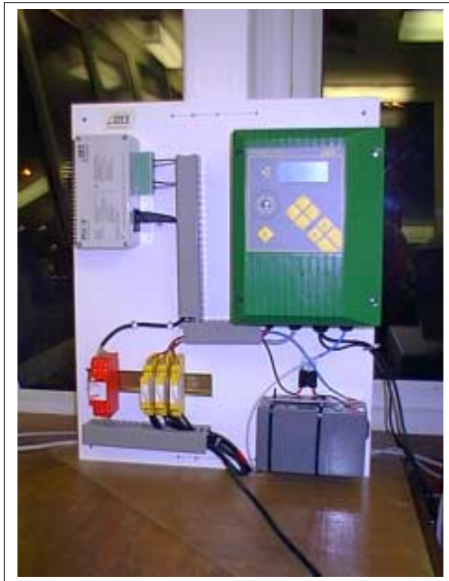
Plate 2.1 Killybegs Nimbus and Corrosion Sensors
