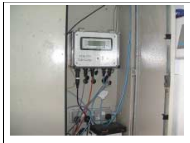
Plate 2.22 Gauge Control Box
