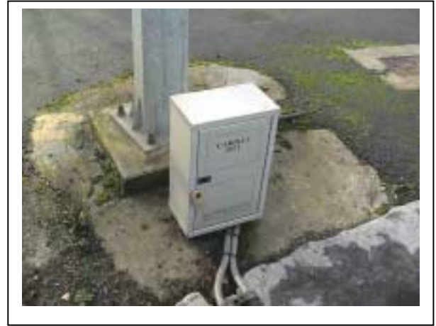
Plate 2.16 Gauge Control Box
