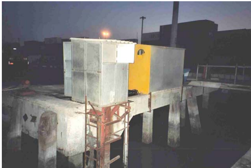
Figure 11. Float gauge (manufactured by the Ott company) in Bushehr.
