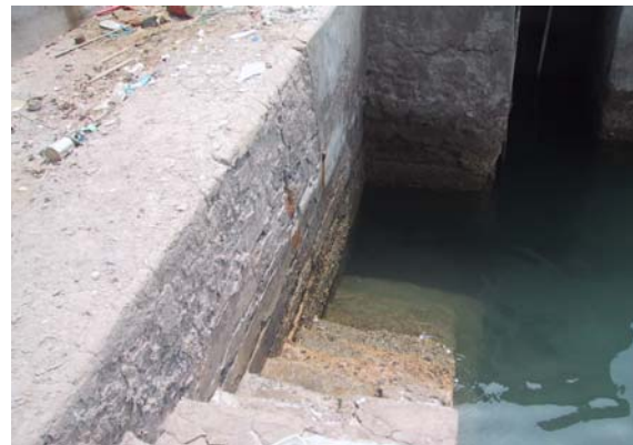
Fig 11. Pilot's Pier Tide Gauge Hut Bench Mark. On vertical left wall above lower step (badly rusting).
