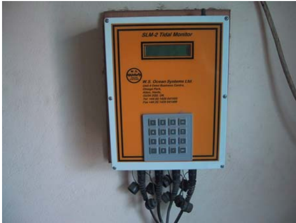
Fig 8. Tide gauge control unit in night watchman's hut.
