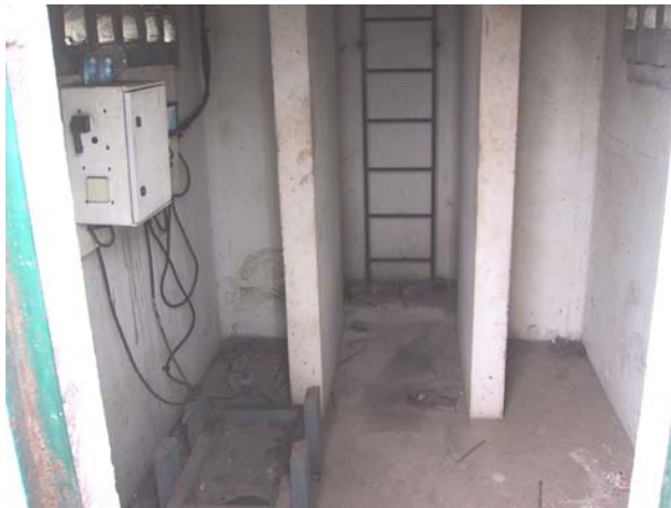
Figure 21. Interior of the navigation tower with electrical junction box and tower ladder.
