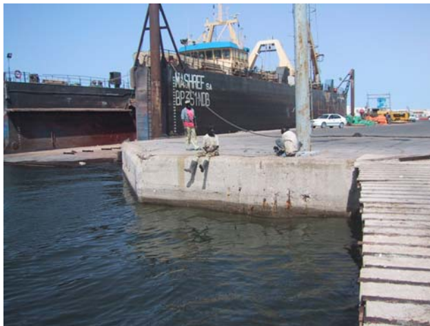
Figure 6. Location 2. Alternative location for a tide gauge at the Southern end of the jetty.
