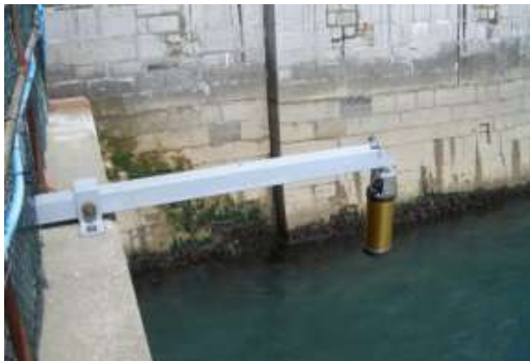
Illustration 2- OTT Kalesto Radar Sensor at Holyhead
