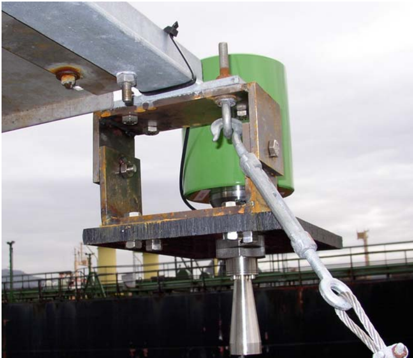
Figure 7 Horn antenna of the SEBA tide gauge.
