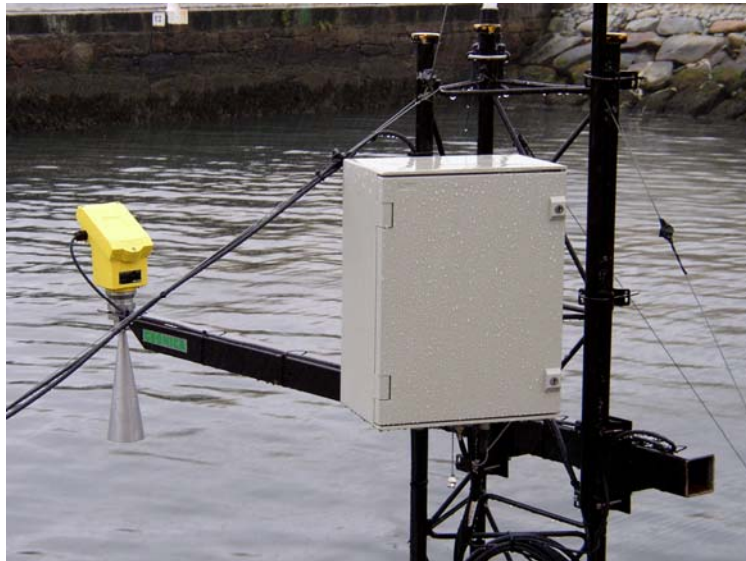
Figure 2 Horn-antenna and box containing the datalogger for the GEONICA system
