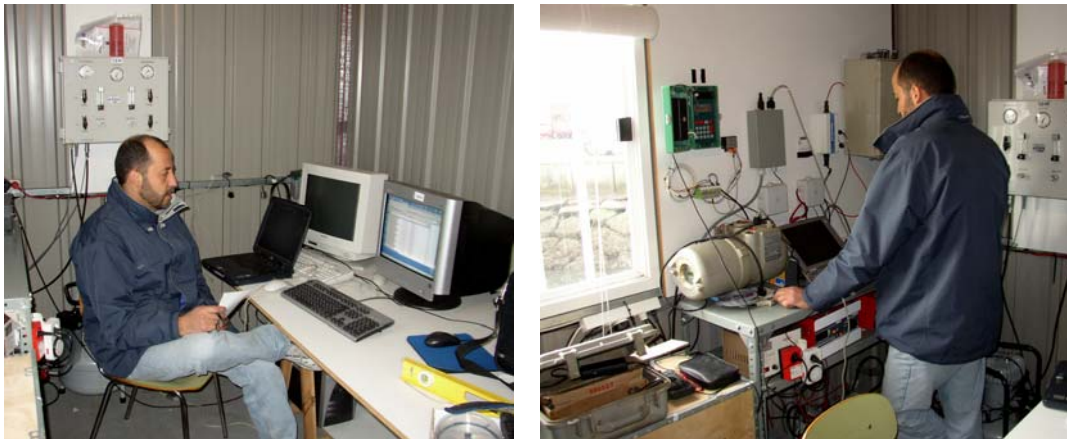
Figure 11 Interior of the hut with the computers and the rest of the electronic devices for the tide gauges.
